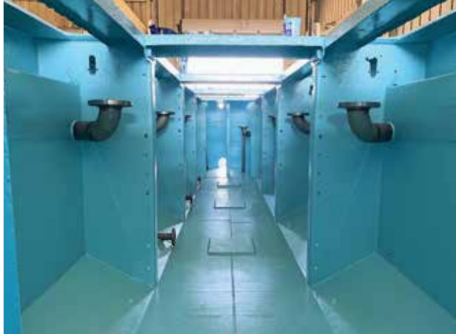
High-solids, edge-retentive coatings help to ensure complete coverage inside pressure vessels featuring pipes, baffle plates and other obstacles.
